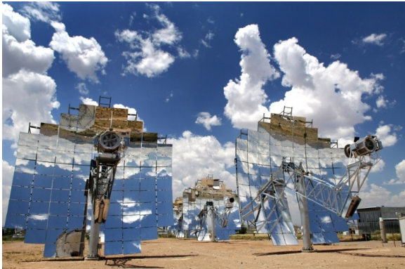
Concentrating solar power system in Albuquerque NM.
