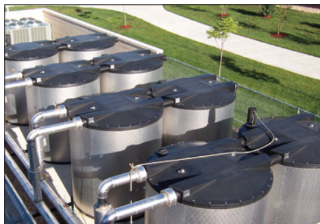
Eight large insulated tanks store ice made during off-peak hours when electrical rates are lower.
