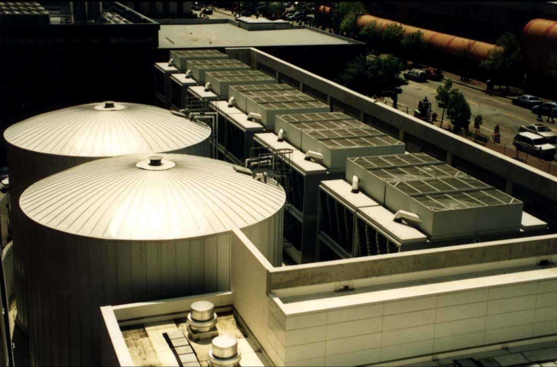
Comfort Link Market Center Chilling Station – Completion (1999)
